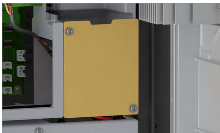
Position of internal fan 2
