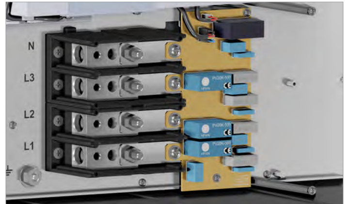
Fig. 4.5: View of type 2 AC surge protection devices with the cover removed
