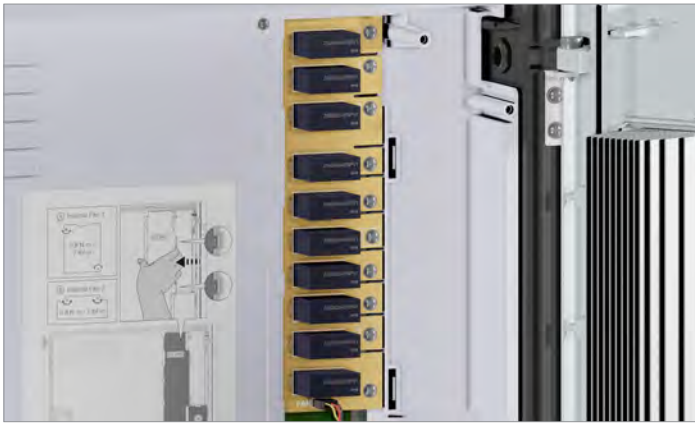
Fig. 4.12: View of the DC surge protection devices with the cover removed
